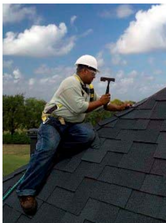
Ben Hernandez of Bent Tree Roof Co. installs Ridglass and Domain Winslow shingles. (Photo by Mark Humphries.)
