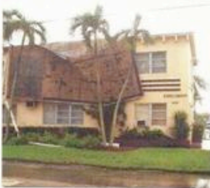
The most severe damage from Hurricane Charley was on buildings that did not have windows and doors protected. (Photos courtesy of Kenneth Kelly, president of Kelly Roofing, Naples, FL.)
