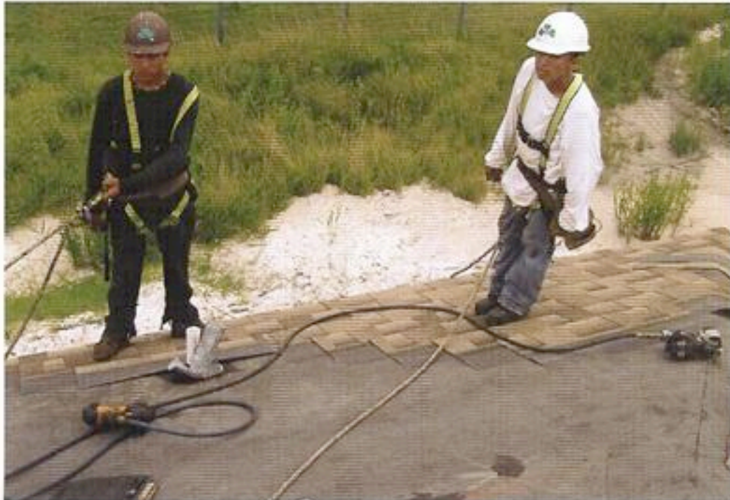
Workers for Kelly Roofing have found that larger-exposure shingles cut down on installation time.
